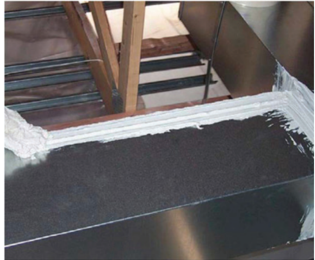
Metal ductwork sealed with mastic.
