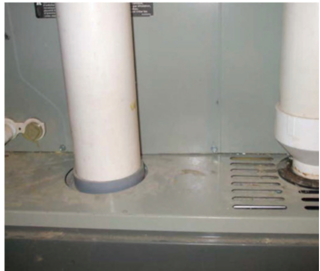
Air handler sealed with silicone caulk.
