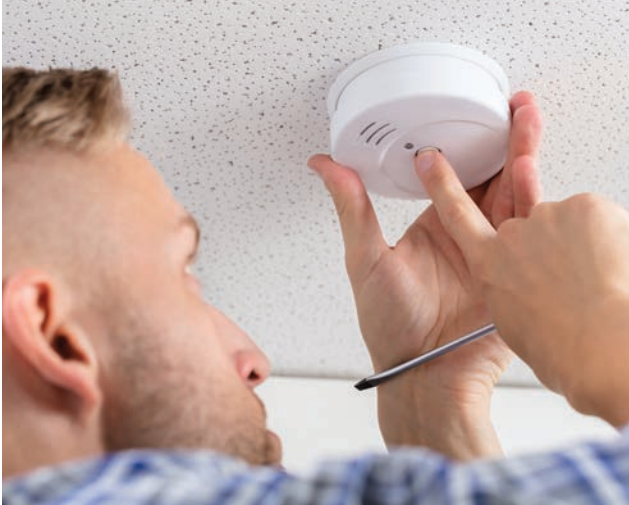
Replace batteries in carbon monoxide testers.
