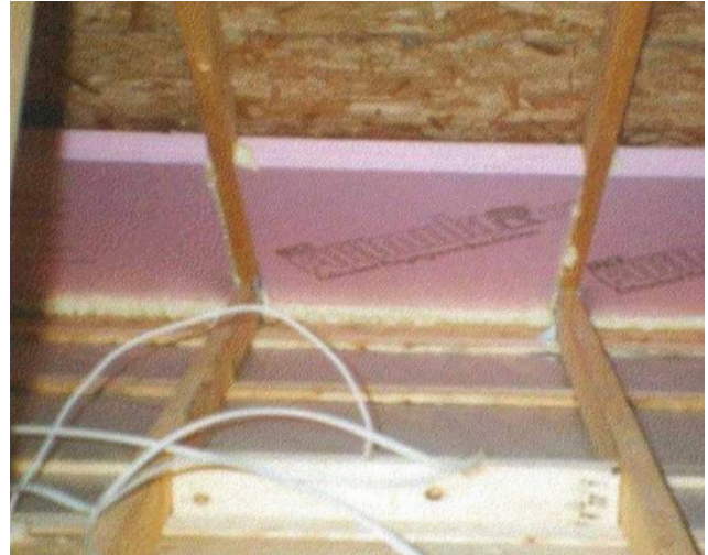
Insulation wind wash baffle.
