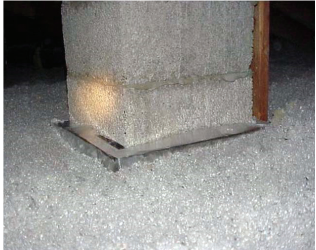
Attic insulation dammed away from chimney.
