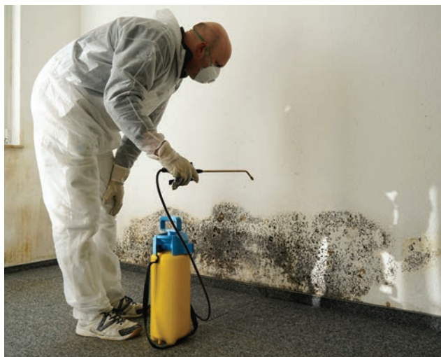
Mold on walls.
