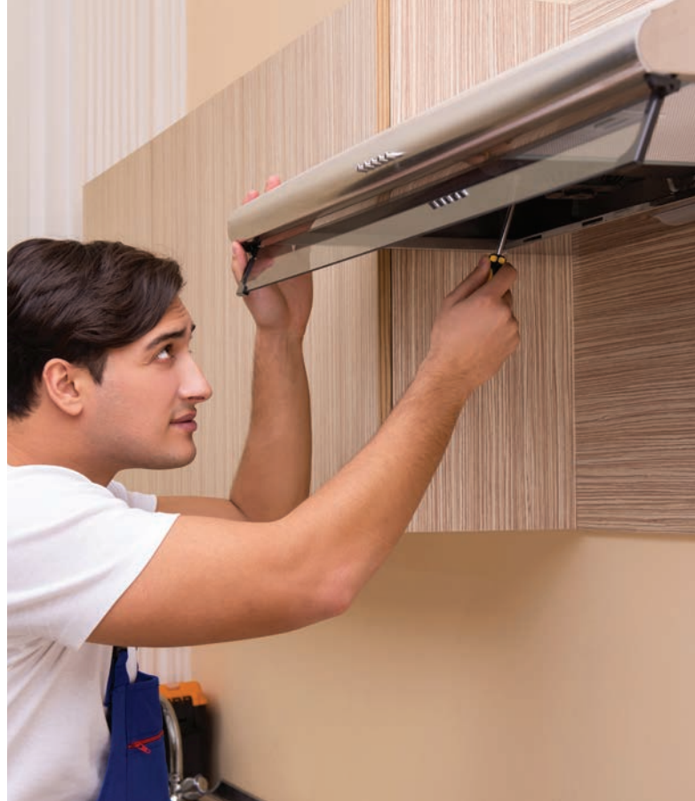
Kitchen exhaust fan.
