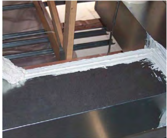
Metal ductwork sealed with mastic.
