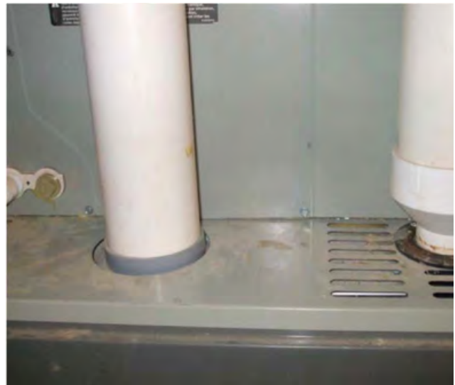
Air handler sealed with silicone caulk.
