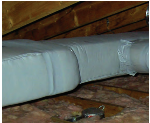
Sealed vapor retarder on attic ductwork.
