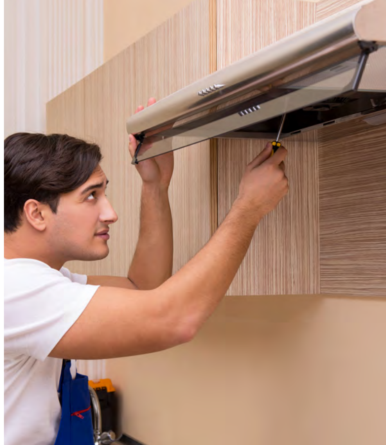
Kitchen exhaust fan.
