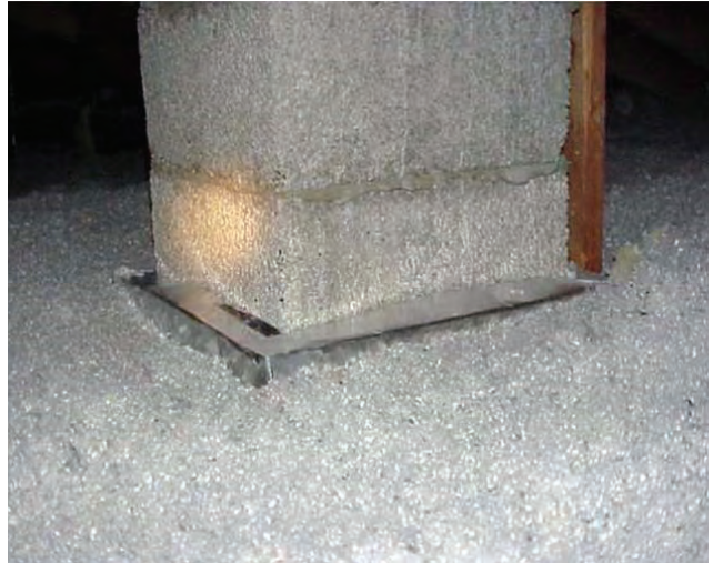
Attic insulation dammed away from chimney.
