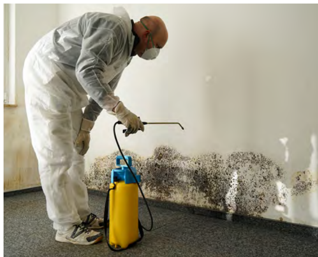
Mold on walls.
