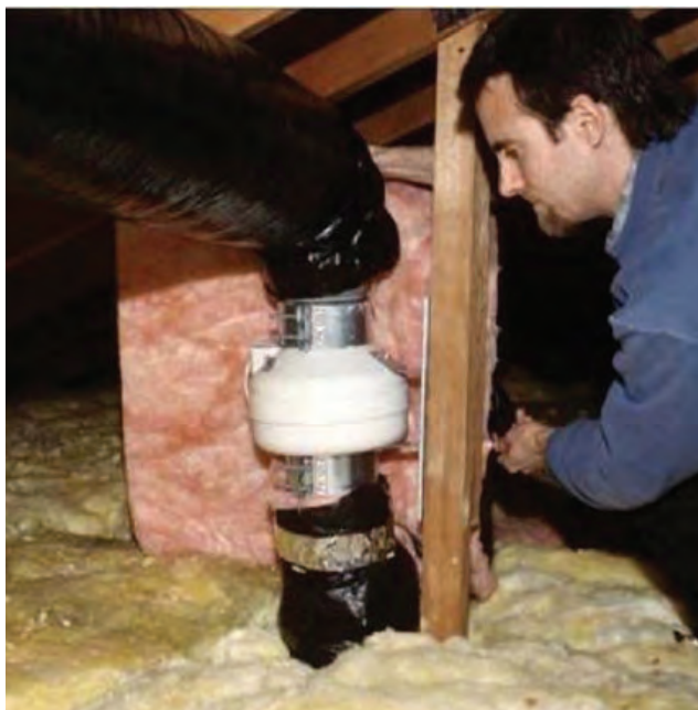
In-line exhaust fan ventilation.
